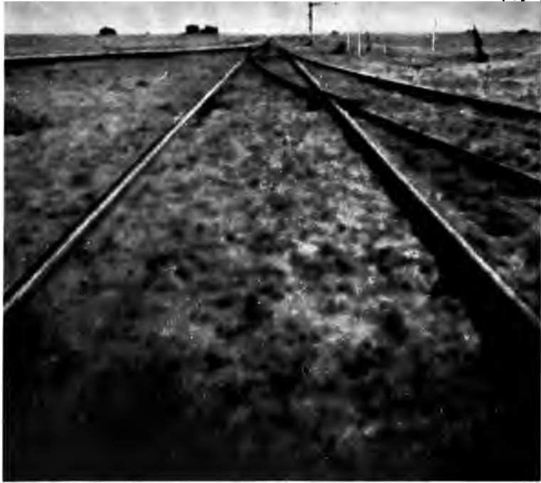
THE NORTHERN END OF THE "TRIANGLE" AT NO. 6 STATION IN THE ABU HAMED DESERT.
